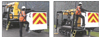
Safe access to bucket from ground or Morooka chassis
