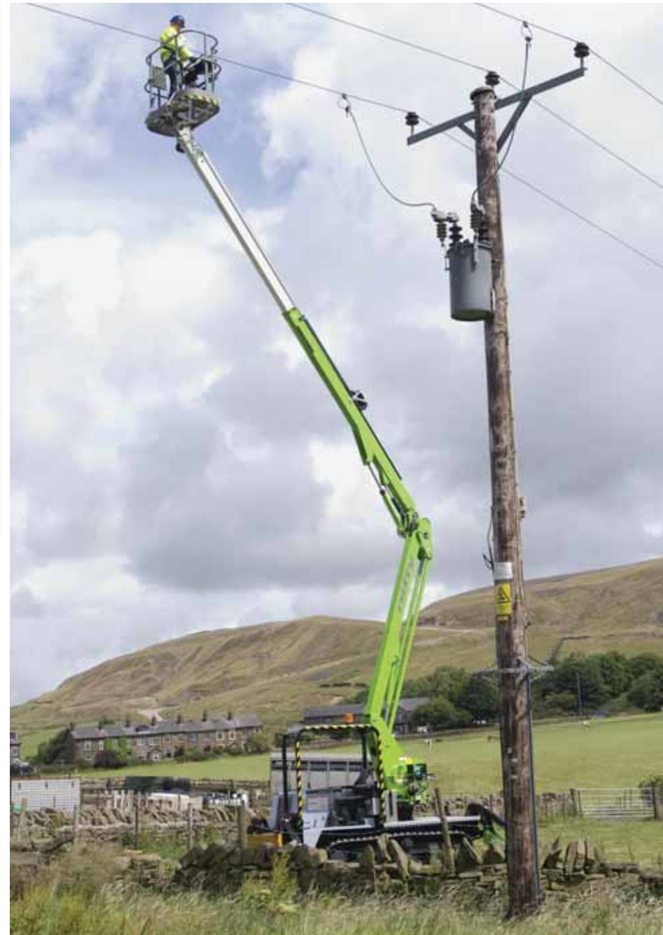
This Picture and Above: Insulated boom sections are available for work on power lines if required, with a wide working envelope from this go-anywhere platform.
